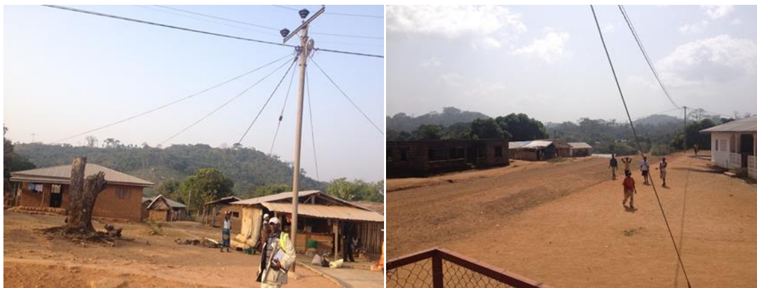
Low Voltage distribution system on poles
