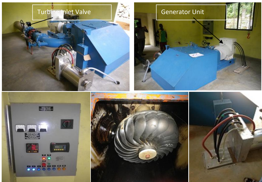
Turbine inlet valve, generating unit, Turgo Turbine, panel, protection panel, ballast load, etc.,
