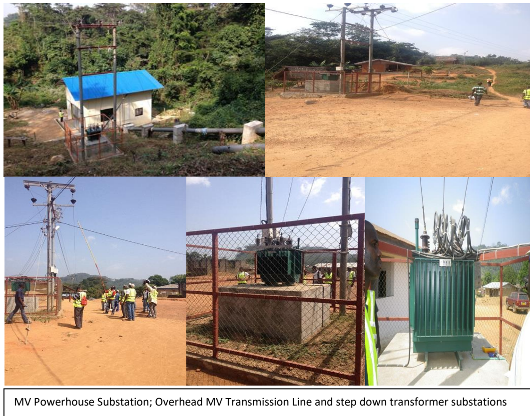
Figure 9: MV Powerhouse Substation; Single Circuit Overhead MV Transmission Line and step down transformer substations
